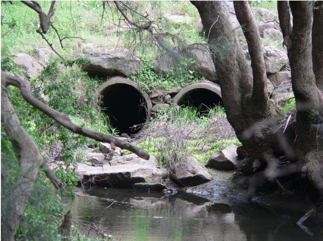
Plate 9: Levee Option 1 - Close up view of stormwater outlets at approximate Ch. 80m.
