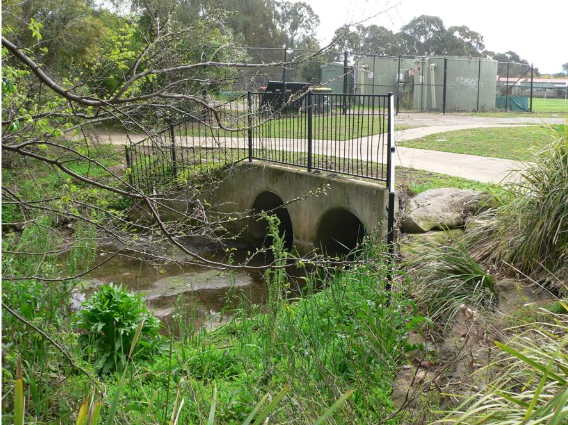
Plate 16: Channelisation Option 2 - View of the stormwater outlet to the north of the channel, at approximate Ch. 240m on the alignment.
