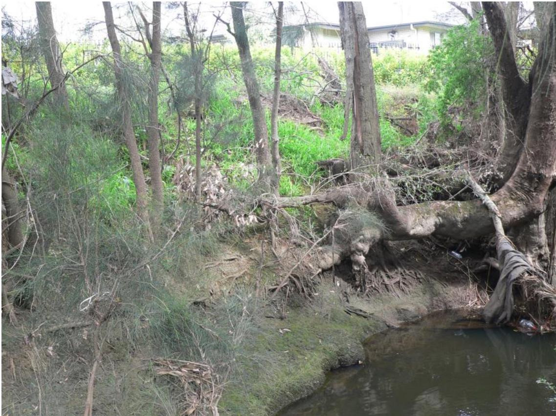
Plate 5: Levee Option 1 - View of the moderately steep bank leading to the creek. Top of the bank is in close proximity to the properties.
