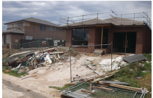
No erosion and sediment controls in place, resulting in sediment running off into the gutter.
