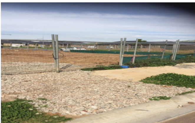
Well maintained building site, stabilised driveway, sediment fencing in place around low point.
