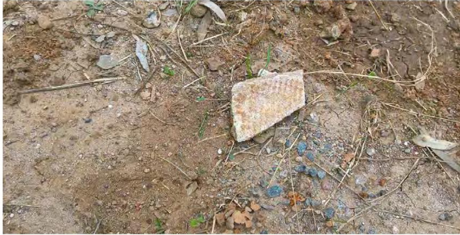
Photograph 9 - Fragment of ACM on surface soils in north eastern portion of site.
