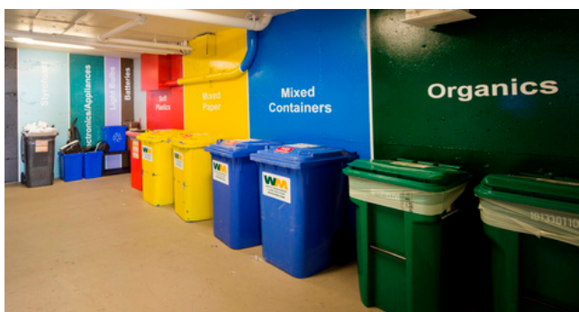
Figure 2-120 Well designed, easily accessible and clean waste and recycling rooms improve the collection and management of household waste
