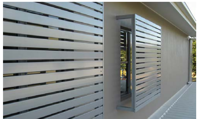
Figure 2-70 Poorly executed privacy screens. These block sunlight and daylight to windows.
