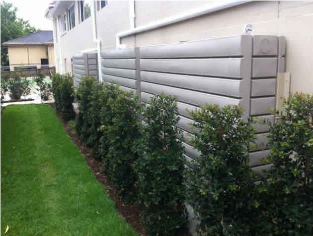
Figure 2-116 Integrate rainwater tanks into the landscape
