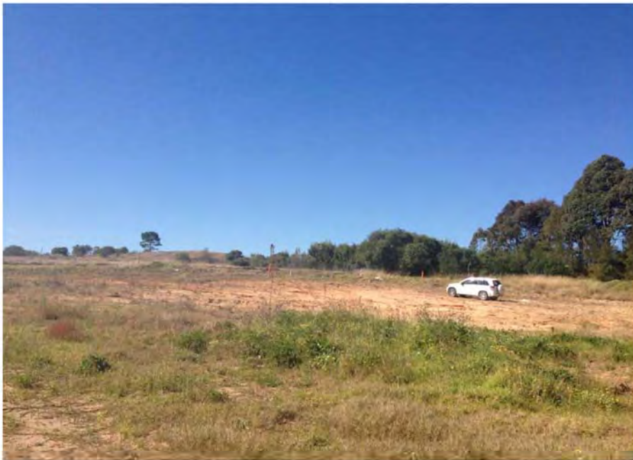
Photo 2 - western end of the proposed haulage road showing cleared road corridor and remnant/regrowth and planted vegetation.
