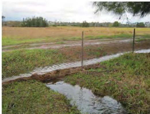
Photo 12: Discharge Point Towards Narrelan Creek at the Southern Boundary of 9 The Meadows
