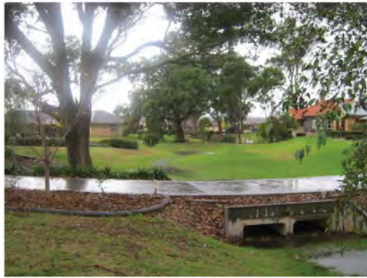
Photo 8: Overland Flowpath Through 10 and 12 The Outlook (Looking Downstream)
