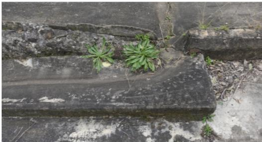
Image 2 – Detail of the south end of the main slab with the drainage channel. Note: this feature would be retained beneath the proposed structure.
